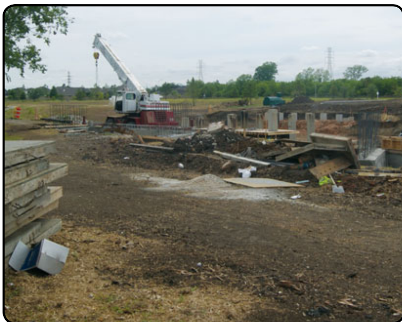
Construction crews working on the Hughes Road/Barry Rose expansion into Pearland received an unexpected day off Wednesday, June 22, due to rainfall. It was the first rain day the workers have had since the project began in early May. The South Belt community was in dire need of the moisture, as the area had not received any significant rainfall in more than 90 days.
