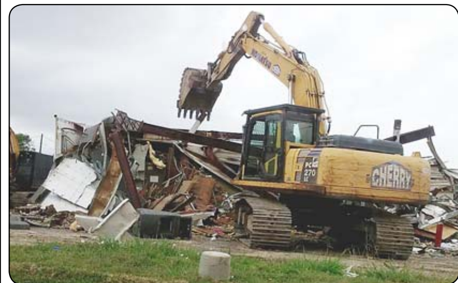
The convenience store at the intersection of Beamer and Hughes Road was demolished Monday, April 10, following a lengthy police investigation. The store had shuttered its doors weeks prior to the demolition. Officials from the Harris County Precinct 2 Constable's office allege the store, along with two others in the area, was part of a citywide ring that sold the synthetic marijuana product Kush.
