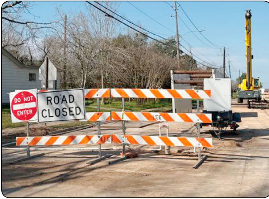
The South Belt community is currently inundated with construction projects, with multiple endeavors simultaneously taking place on some of the area's most busy roads. The majority of the projects involve an extensive Houston Public Works undertaking to consolidate three local wastewater treatment plants, decommissioning two in the process. Crews are shown above working on Fuqua near Kingspoint, where the Easthaven Wastewater Treatment Plant is being diverted to the city's Southeast Wastewater Treatment Plant on Genoa Red Bluff.
